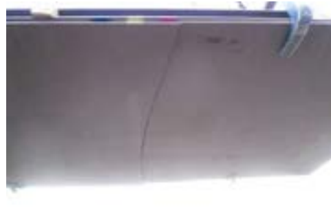
Example of a three-point lift with a crack as a result.
